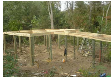
Construction has begun on the River Landing camping platform. This will be available for users of the Roanoke River Paddle Trail.
